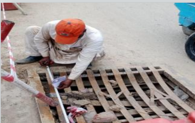
Manholes coverage in Swat
