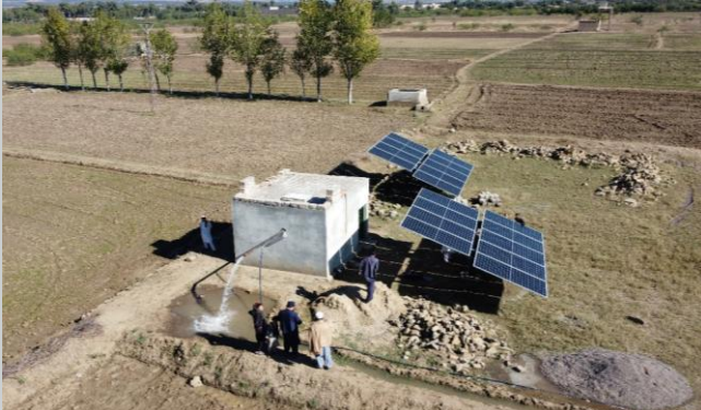
Solarized Tubewell - Hangu
